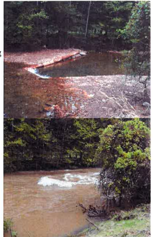
Fair Crossvane at installation (top) and during high water (bottom)
